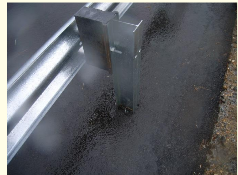
Typical guardrail installation in Georgia (driving through a thin layer of asphalt)
